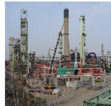
Neste Oil refinery (vegetable oil) in Porvoo, Finland
